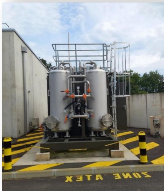
Grid Access © Arol Energy
